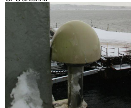
Figure 8. Cracking to outer casing of a GPS antenna
