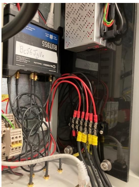
Figure 50 Battery and solar terminal block.
