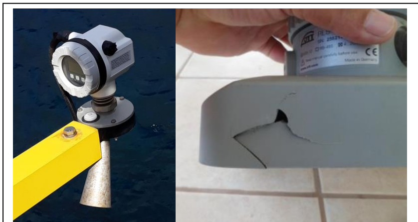
Figure 10. Damaged radar horn (left) and cracked sensor housing (right)
