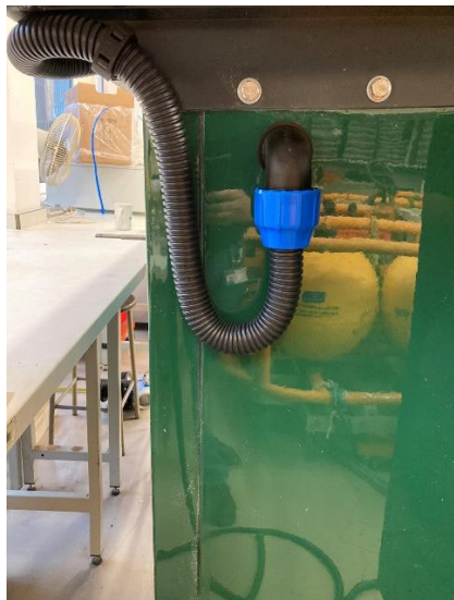
Figure 15 Solar panel cable conduit.
