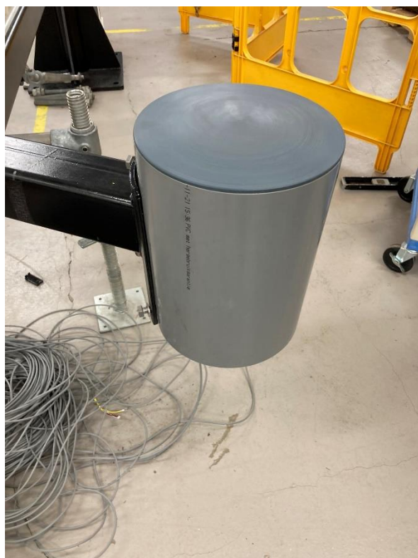
Figure 51 Radar protective cover.
