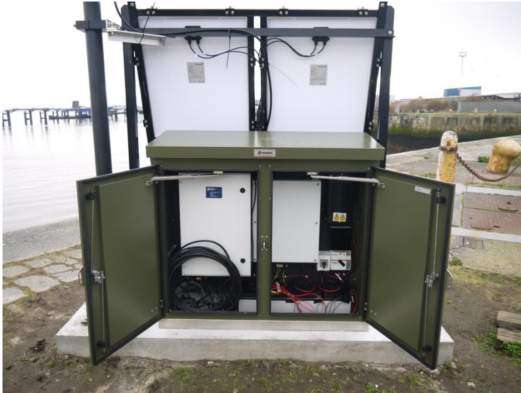
Figure 5 Photo showing the solar panel frame, equipment cabinet and Yagi antenna at Alfred Dock.
