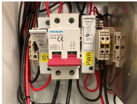
Figure 30 Open the fused circuit breakers.
