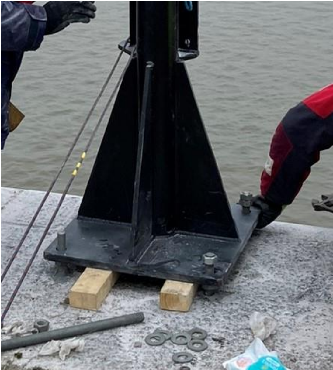
Figure 12 GNSS mast anchor bolts.
