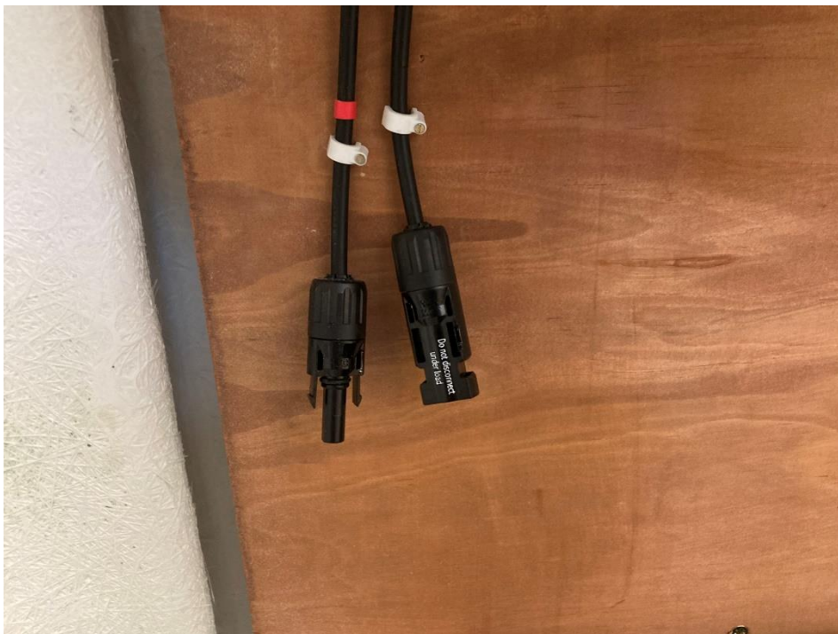
Figure 24 Solar panel connector
