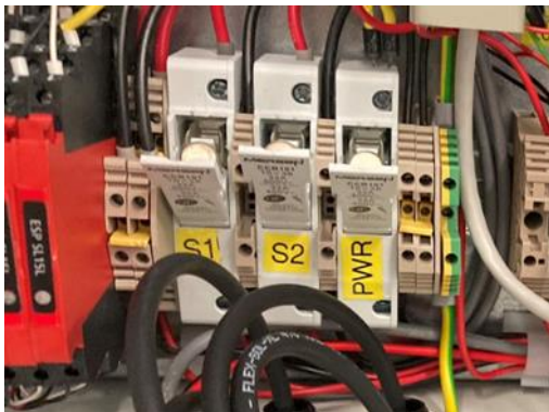
Figure 29 Logger enclosure fuses in open position.
