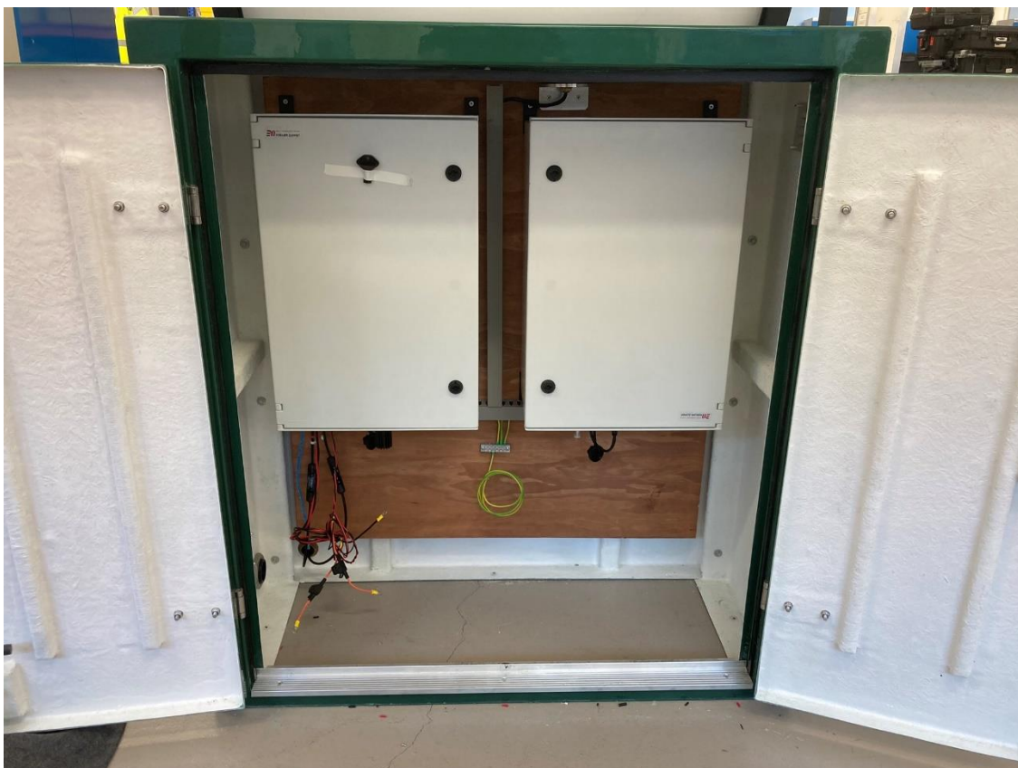
Figure 34 Equipment cabinet showing the logger and GNSS enclosures.
