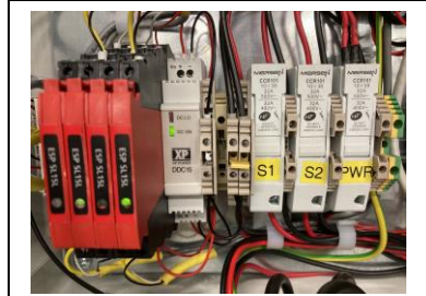
Figure 16. Fuses and surge protectors
