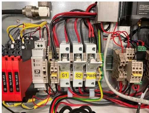
Figure 44 Logger enclosure fuses in open position.
