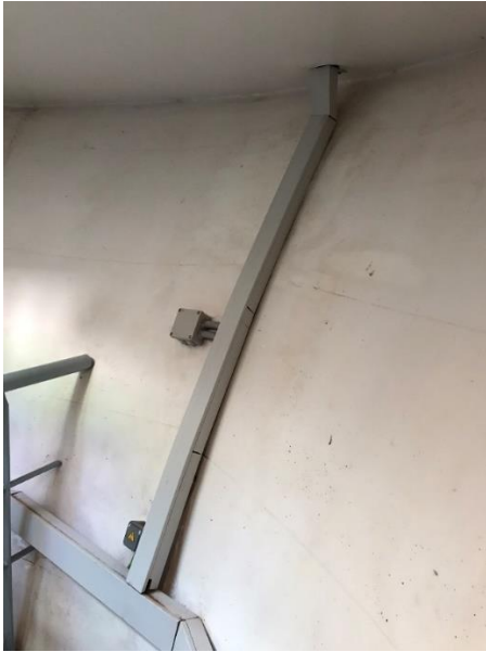
Figure 43 Trunking carrying cables from light platform.
