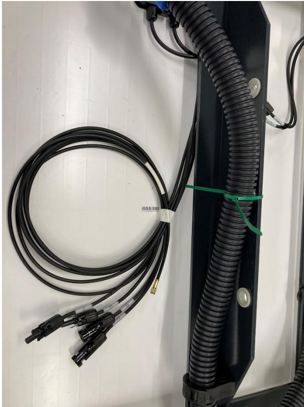
Figure 34 Solar panel cables.
