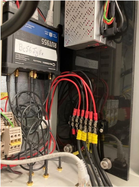
Figure 34 Battery and solar terminal block.
