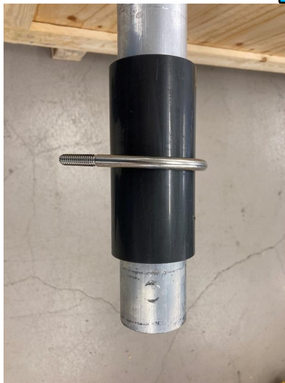
Figure 31 Yagi antenna mast attachment point.
