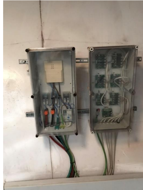
Figure 44 Existing equipment enclosures that will be removed.
