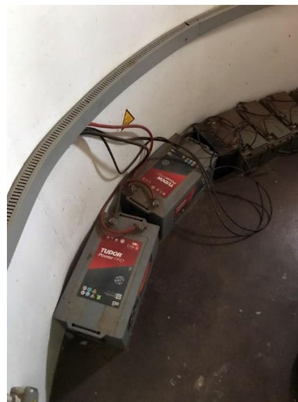
Figure 46 Lighthouse battery bank.
