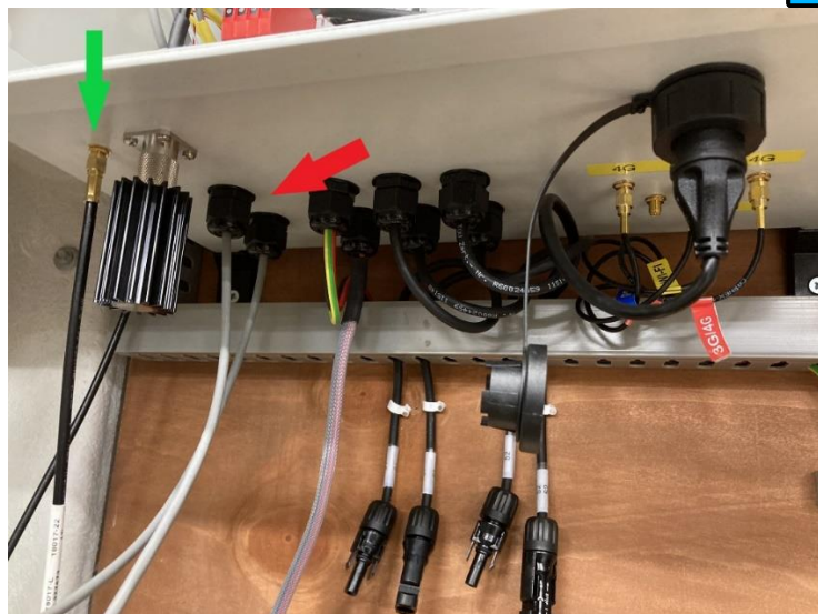
Figure 36 Meteosat Yagi antenna connector and radar cables.
