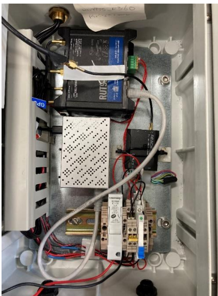
Figure 45 Low cost GNSS.
