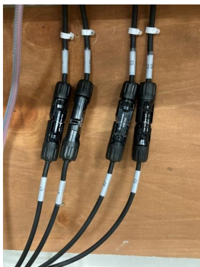
Figure 46 Solar panel leads connected to system.
