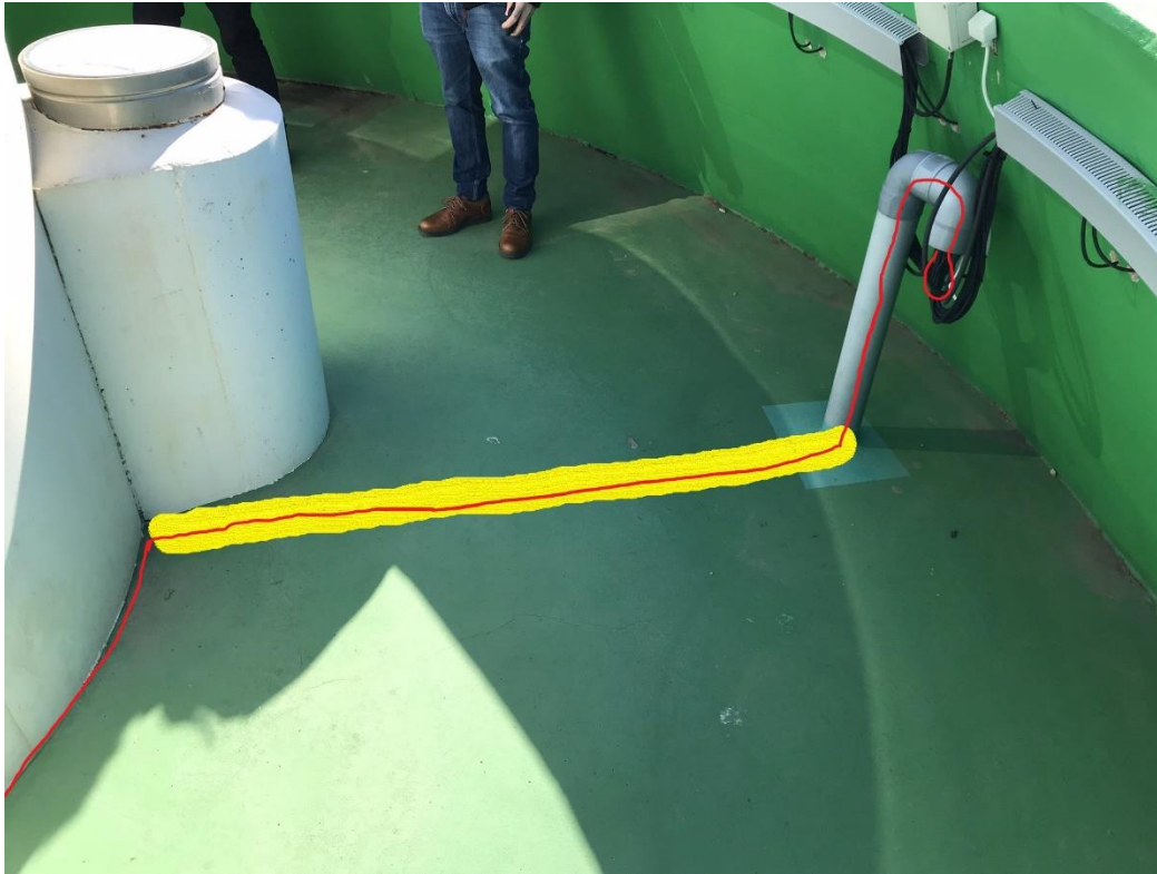
Figure 41 Lighthouse cable access point.
