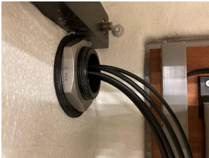
Figure 16 Solar panel cable entry.
