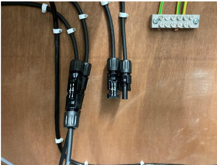
Figure 25 Solar panel connector
