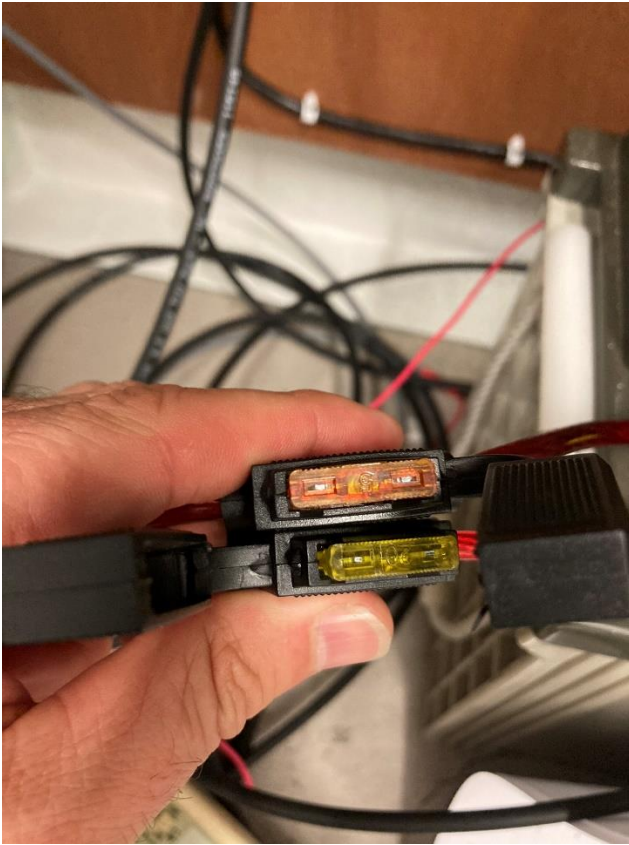
Figure 28 Battery bank blade fuses.
