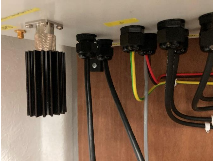
Figure 24 Meteosat Yagi antenna connector and radar cables.
