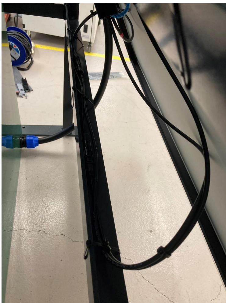
Figure 11 Rear of solar panel showing conduit access to cabinet for solar panel cables.
