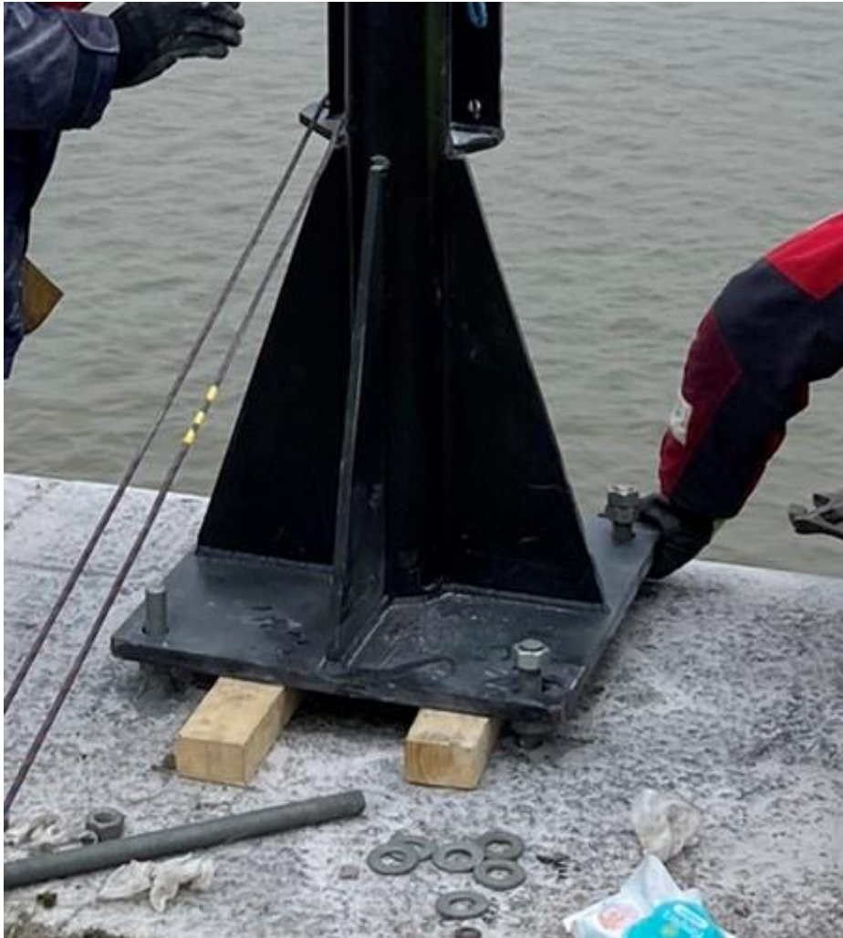
Figure 9 GNSS mast anchor bolts.
